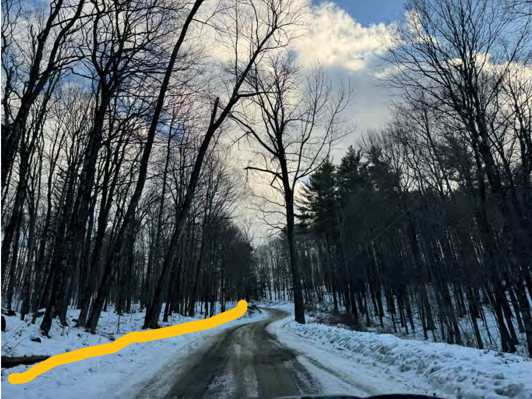
135500 before 1 - widen road 2-4ft and install stone line ditch on left side going uphill
