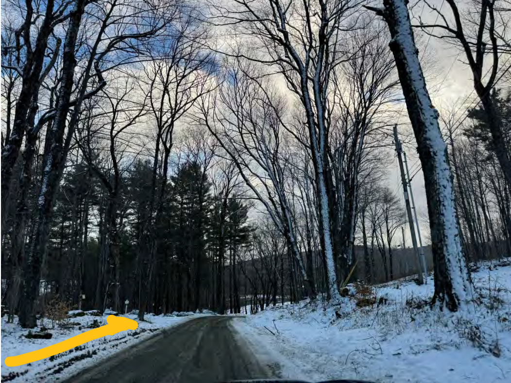
135498 before 1 - widen road 2-4ft and install stone line ditch on left side going uphill
