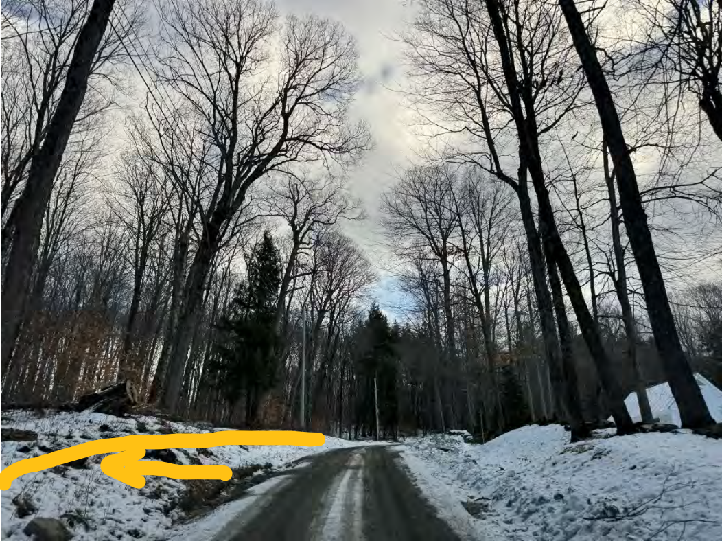
135502 before 1 – widen road 2-4ft and install stone line ditch on left side going uphill
